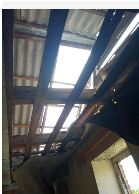
Roof Damage Caused by Heavy Rain and Strong Winds in Akhmeta
